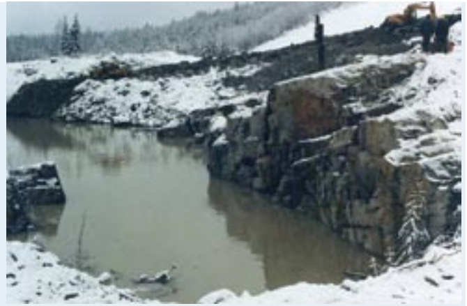
Figure 3. Filling of the Paukkajanvaara mine in Eno, 1993. The Finnish Centre for Radiation and Nuclear Safety gave the certificate of the accomplished environmental restoration of the mine area to the landowner in 2001 /13/.
