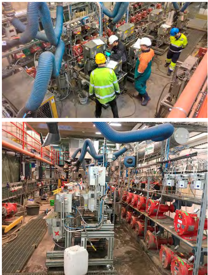
Figure 2. OMS Pilot plant
