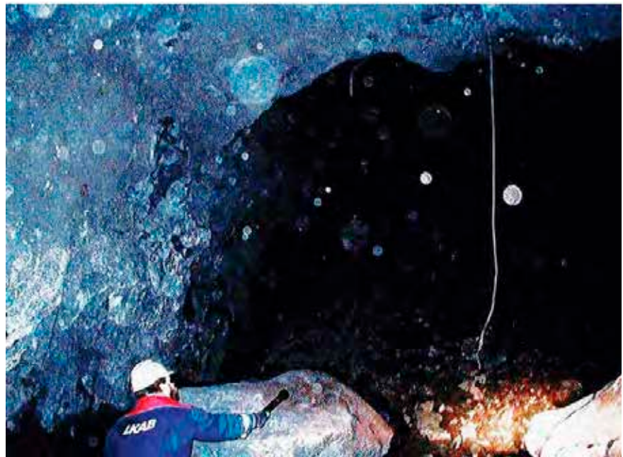
Fig. 1. A large empty room formed due to hanging roof in sublevel caving [1].
